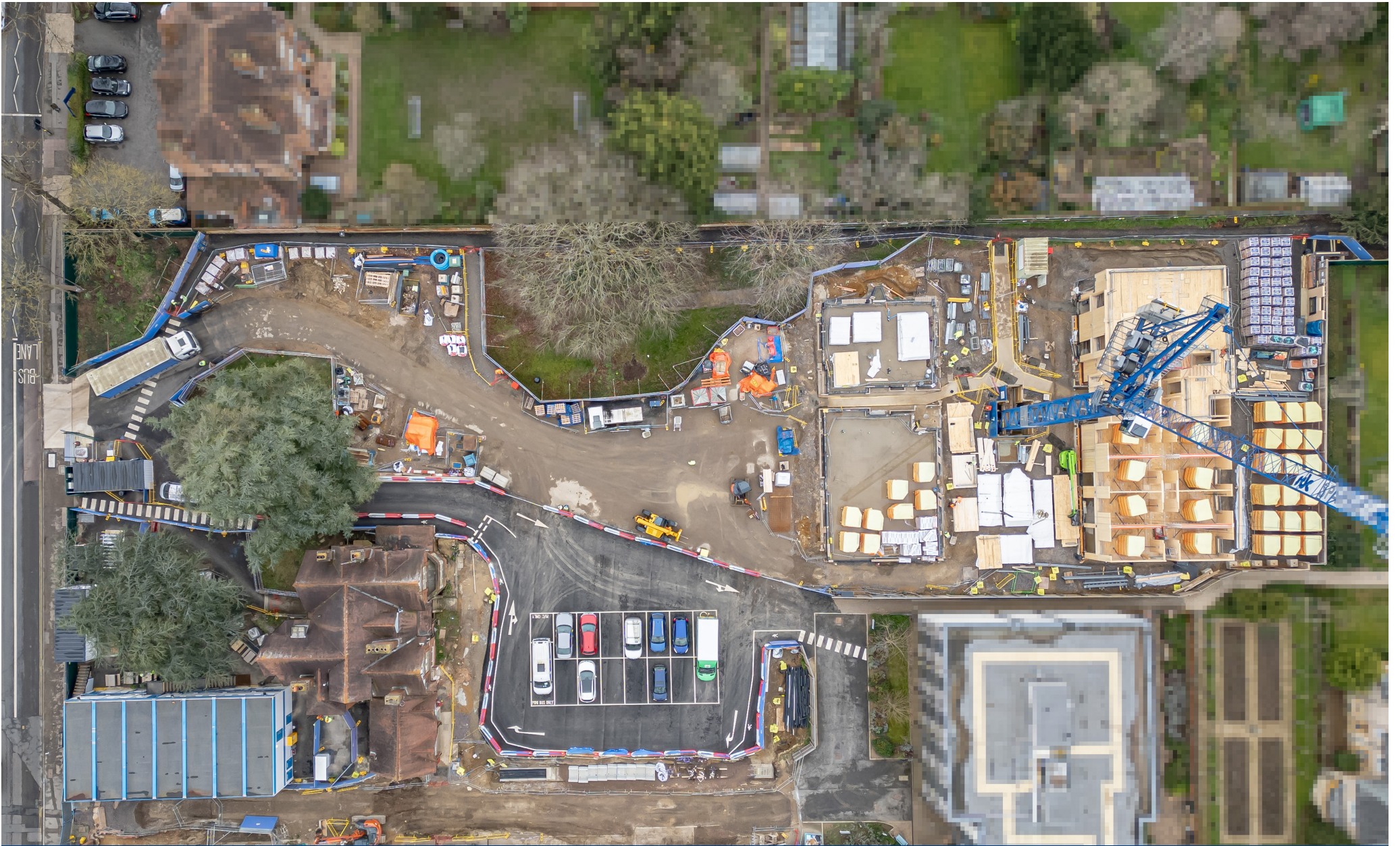
This was how the site looked in April with a temporary car park installed for the Fairfield Residential Home to use whilst their access road was removed.
