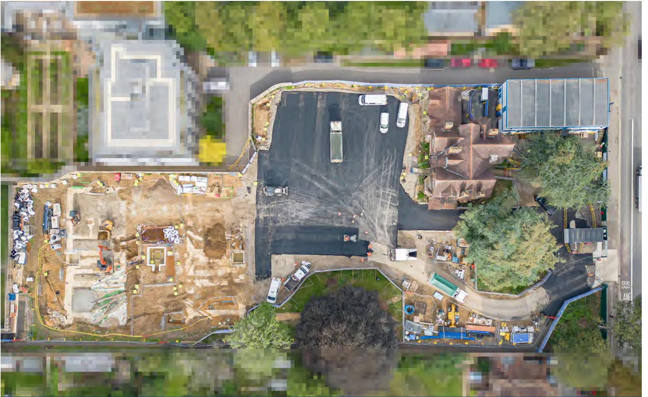
A temporary car park was built for the Fairfield Residential Home to use whilst their main access road was blocked during service installations.
