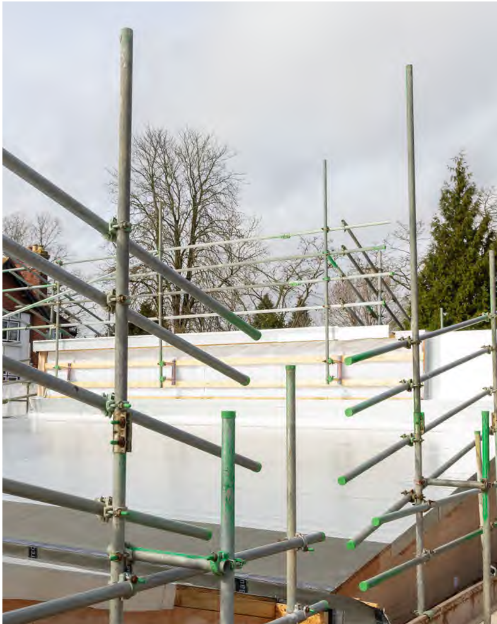
The timber roof has been added and the first roof layer fitted which now makes this watertight allowing the internal finishes to continue.
