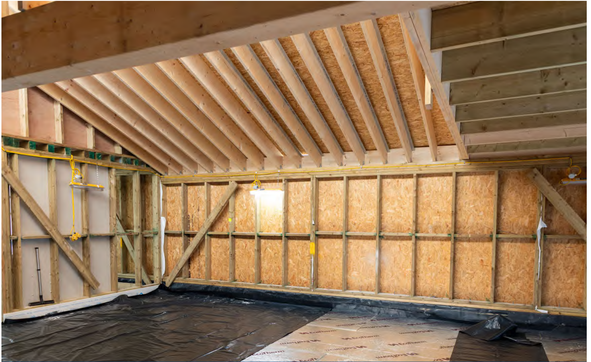
This image shows the 3-5 years room with the flooring insulation installed, prior to the laying of underfloor heating pipework.
